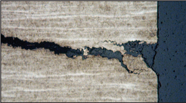
Optical photomicrograph of polished cross section through the cracked axle shaft. 40X
